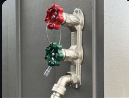
Hose bib, hot and cold
