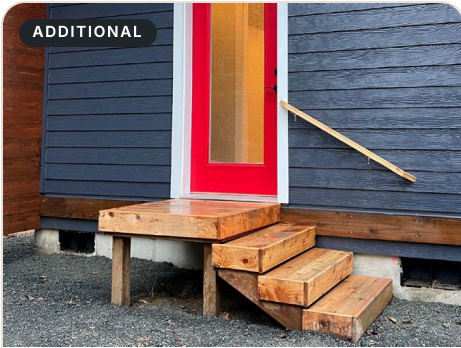
3' x 3' deck The code-minimum landing required for final occupancy.
